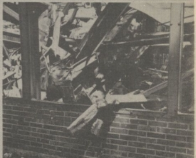
Photo 22 - Allach - Failure of heavy steel structure, bldg 2011. Bolted joints failed.
