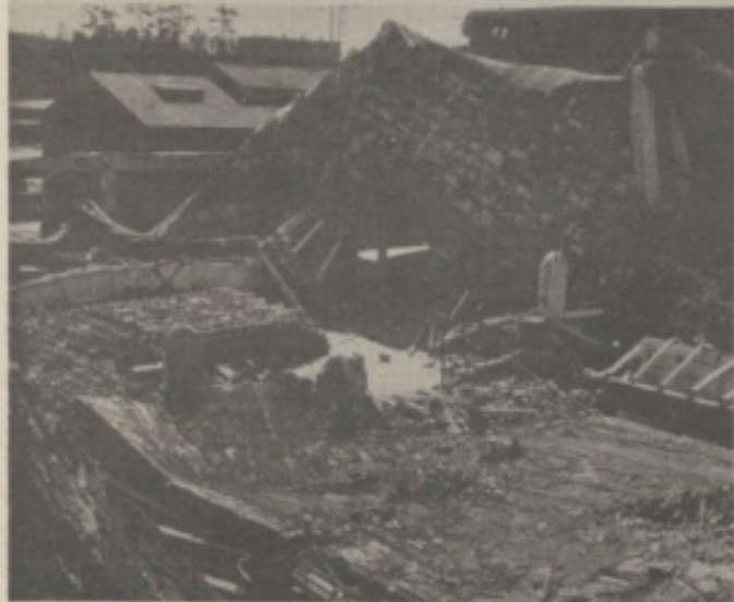
Photo 21 - Allach - Spreading collapse, light reinforcing in column.
