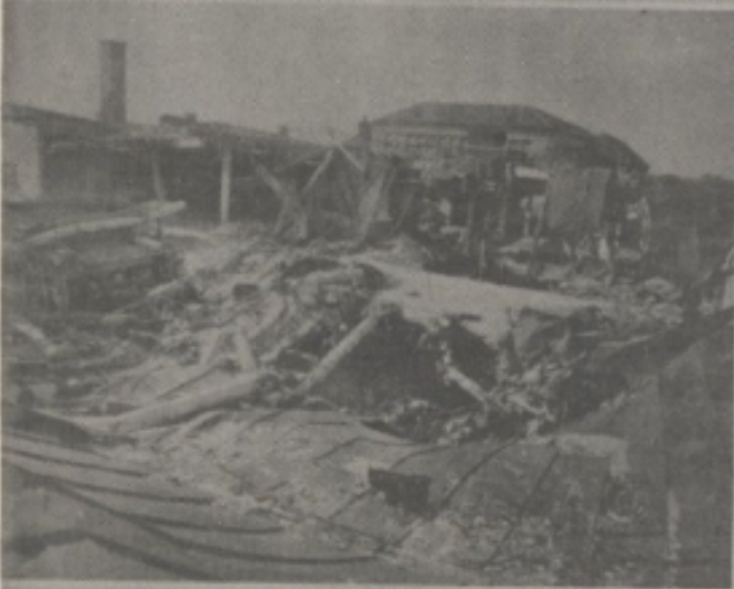
Photo 13 - Oberwiesenfeld - Complete collapse of lightly reinforced concrete structure. Result of three bomb strikes.
