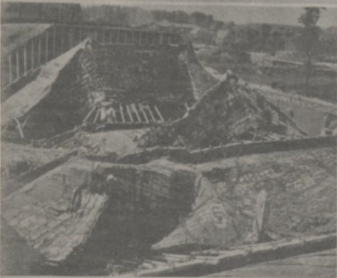
Photo 15 - Allach - Type of failure of lightly reinforced concrete. Bldg 2003.
