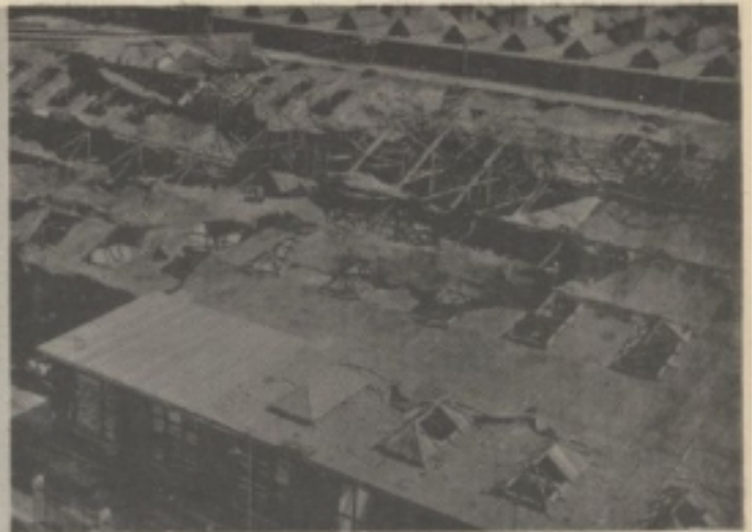
Photo 18 - Oberwiesefeld - Light steel structure destroyed by fire.
