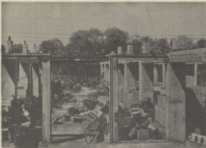
Photo 17 - Allach - Packing bldg destroyed by fire. Debris had been cleaned up.
