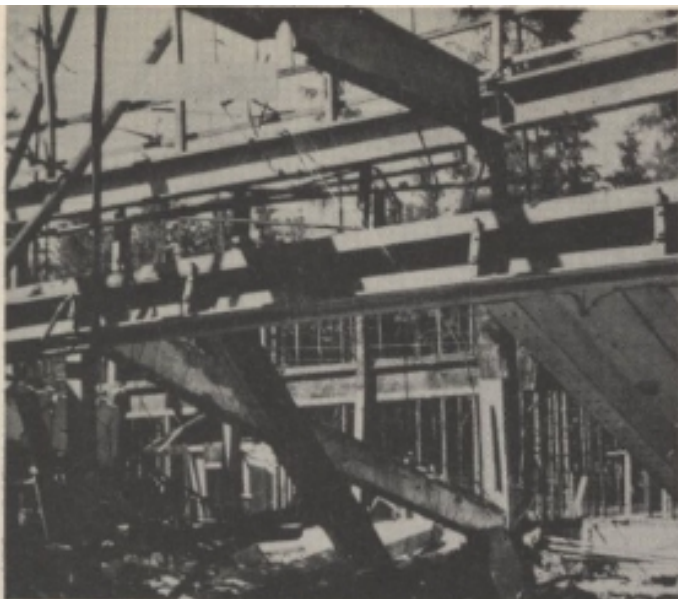
Photo 23 - Allach - Failure of heavy steel structure, bldg 2010. Bolted sections failed.
