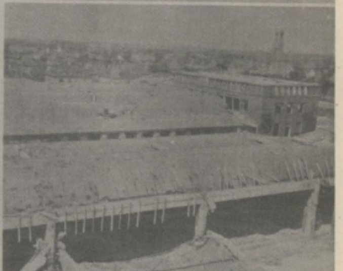
Photo 16 - Oberwiesenfeld - Failure due to blast. New construction.
