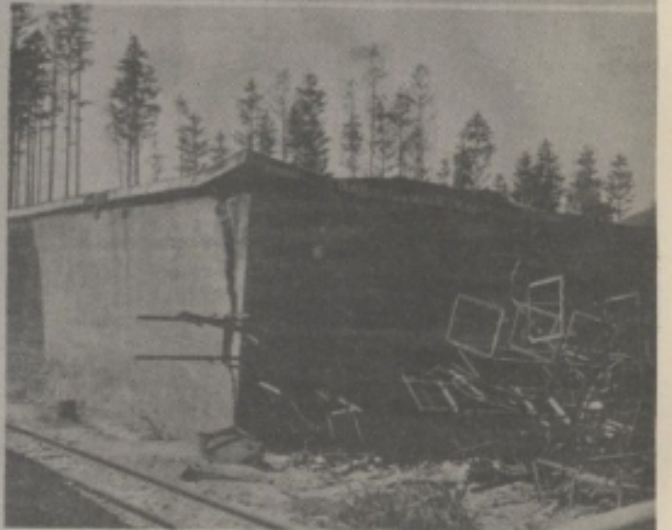
Photo 14 - Allach - Bldg 2091 where storage of light metals burned. Complete destruction of reinforced concrete bldg.
